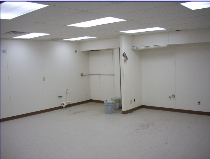
Large production/office area with water and three-phase electric.
