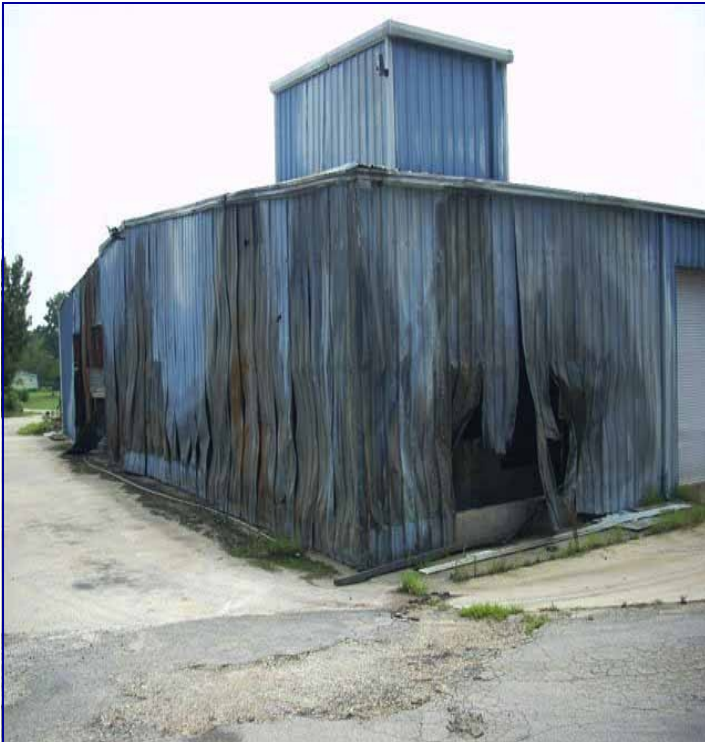
11,200 s.f. main building showing fire damage.
