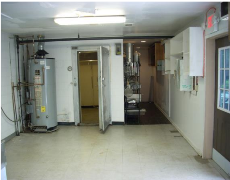
One of two refrigeration/freezers units
